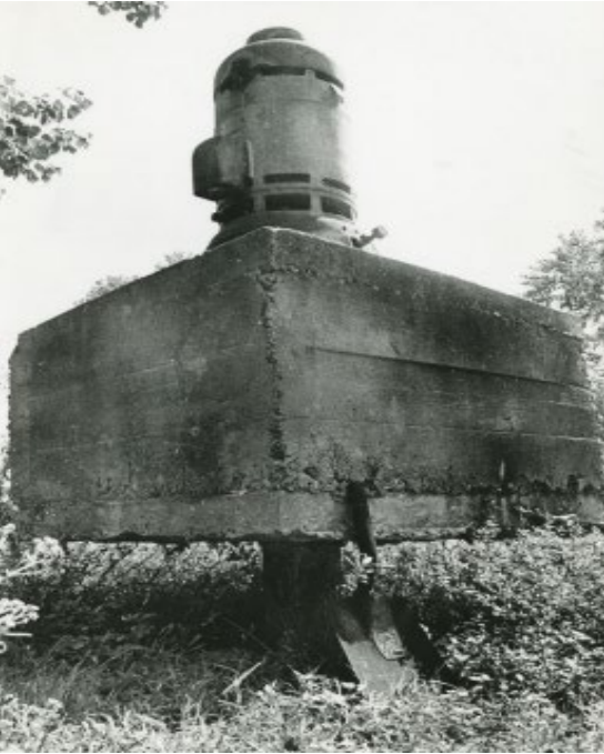
Groundwater well with casing exposed
