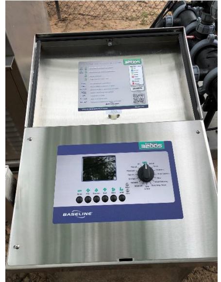
Image 1. Baseline 3200 Smart Controllers at one of the pump stations.
