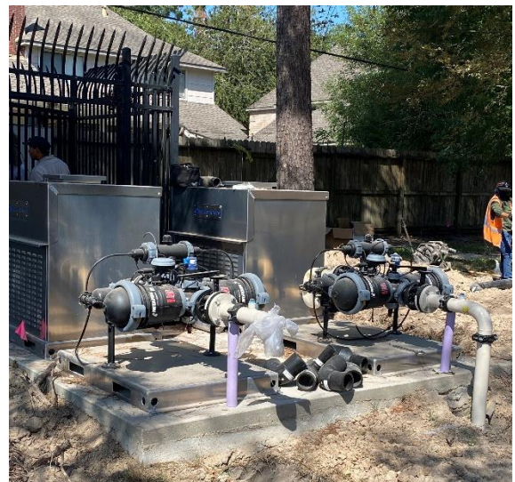
Image 2. Booster pump installation at Bill Lloyd Park.
