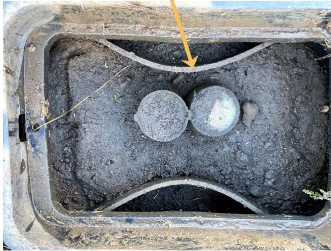
Figure 9: Meter Boxes Filled with Dirt or Debris
