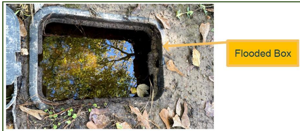
Figure 6: Flooded Meter Box
