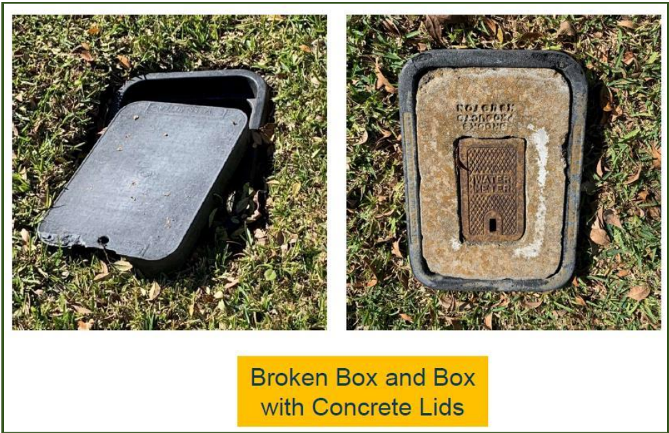
Figure 8: Broken Meter Box / Missing Lids
