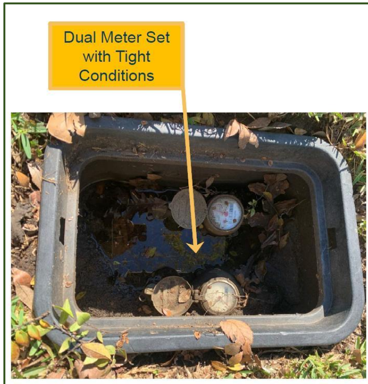
Figure 7: Tight Conditions in Meter Box
